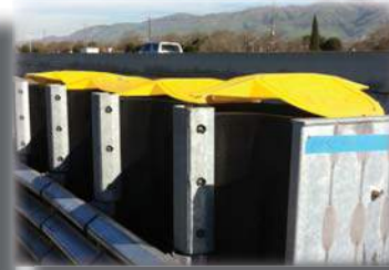
Raised module covers indicate impact
