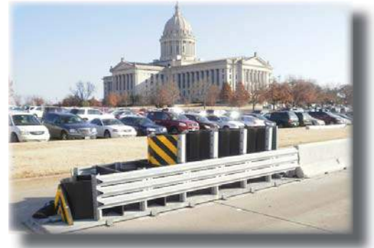
Temporary Compressor® Installation near Oklahoma State Capitol
