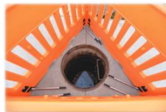
Protect Pedestrians From Work Zone Hazards
